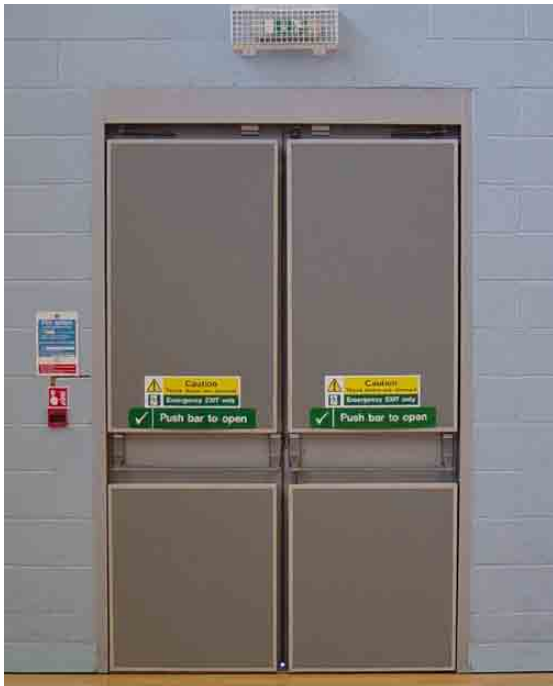
Sports hall walls should be detailed for safety and without hazardous projections. Flush surfaces should extend to 2.0 m minimum, preferably to 2.7 m above floor.
