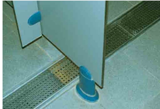
Floor channels with bucket gullies and lift-off grilles give effective drainage in shower and other wet areas. They require regular cleaning
