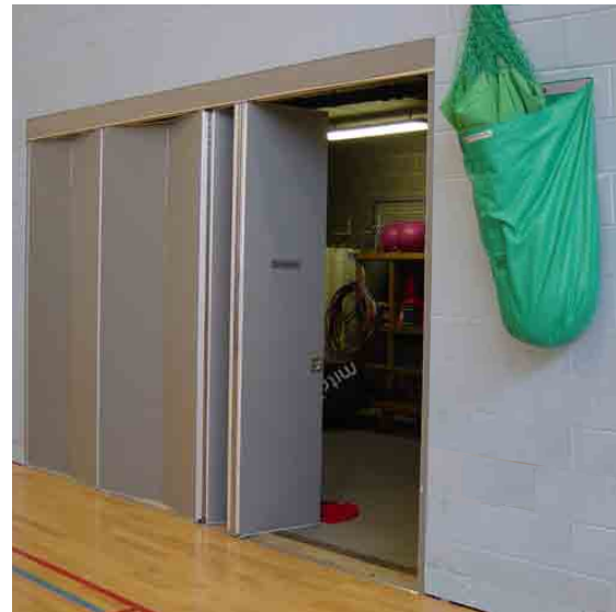
Store doors should be flush detailed, and unless they can only be opened by operators and otherwise kept locked, they should not open out into the sports hall. Doors may need to perform as rebound panels and therefore their construction needs to be robust and safe for users. Net bags should have no projecting fittings/features that could create a hazard and be high enough to not compromise the five-a-side rebound zone (1.21 m).
