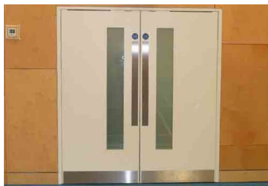
Standard proprietary flush door with a flush viewing panel, opening outwards away from the sports hall
